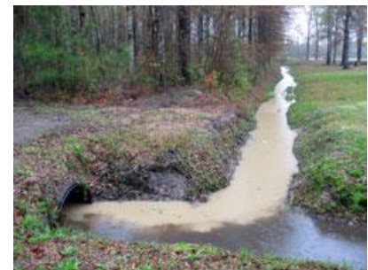
Sediment from construction
